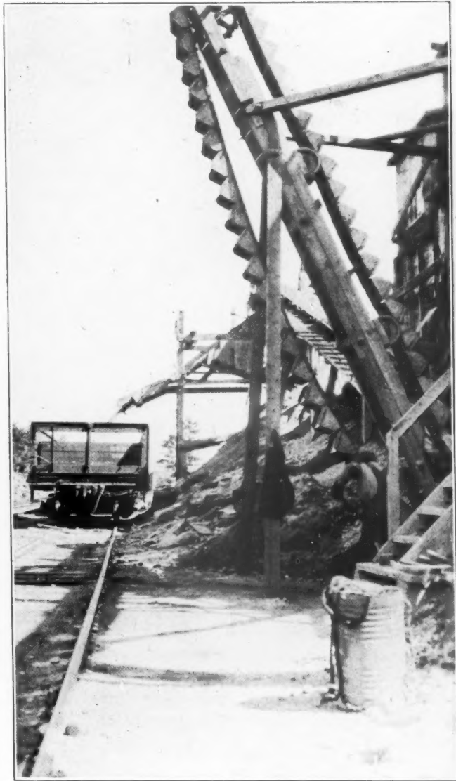
New elevator in foreground for loading freight cars. In the background is the belt conveyor and chute by which cars have been loaded in the past.
